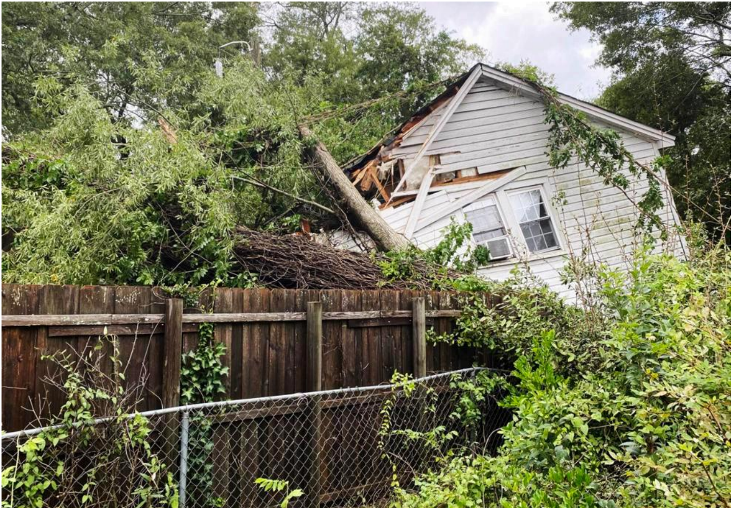
A fallen tree damaged a home in Anderson during Tropical Storm Helene, Sept. 27, 2024.
