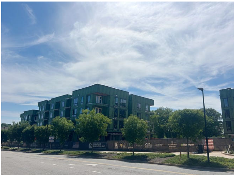
Southernside East, a 93-unit affordable housing complex for seniors, is currently being built near Unity Park. (Ruth Cronin)
